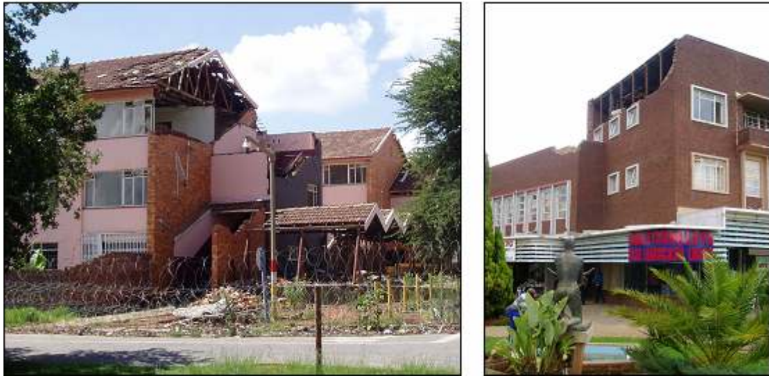
Figure 5. Damage in Stilfontein caused by the ML = 5.3 tremor on 9 March 2005
